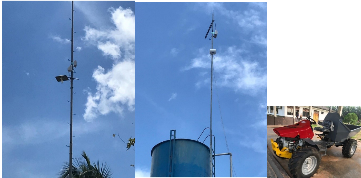
Figure 13: Whizpace devices installed as backbone and last-mile networks
